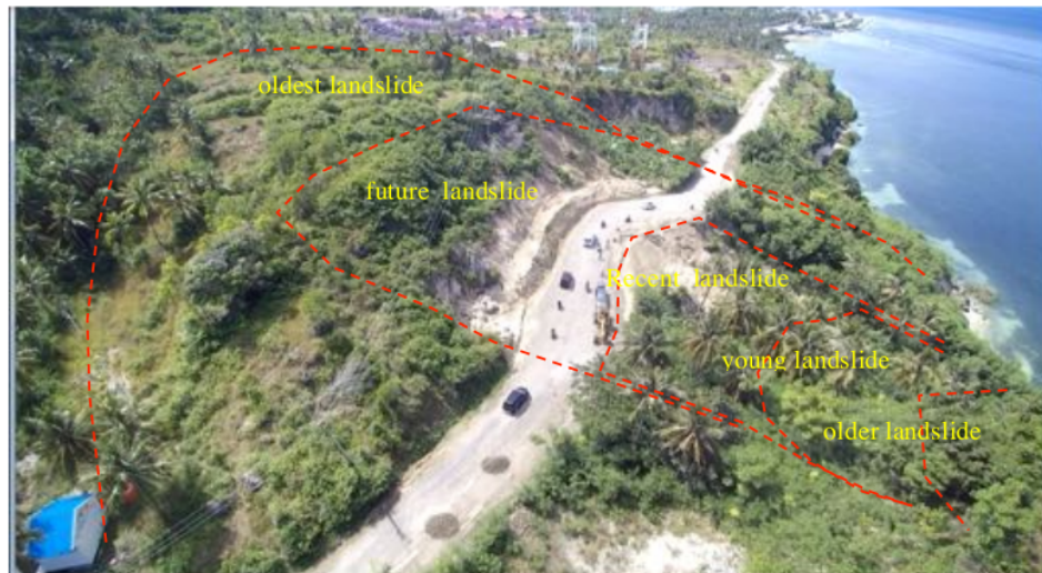
Figure 11. Existing landslide scarps in the landslide areas indicates periodical events of landslide have occurred.
